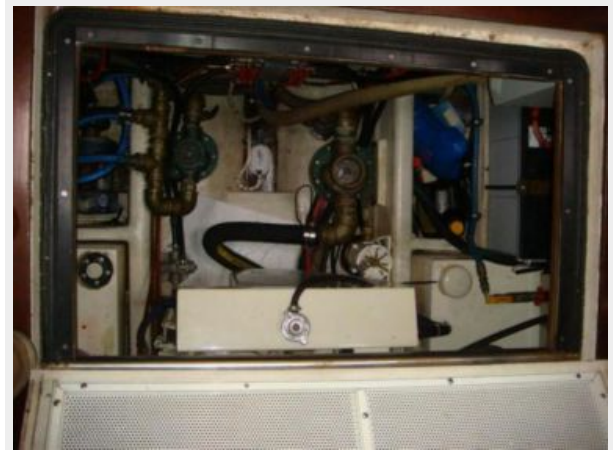
43' Sterling Atlantic engine room access
