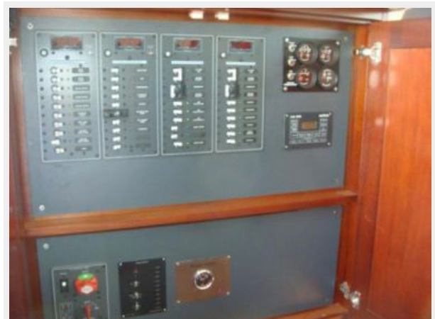
43' Sterling Atlantic electrical panel
