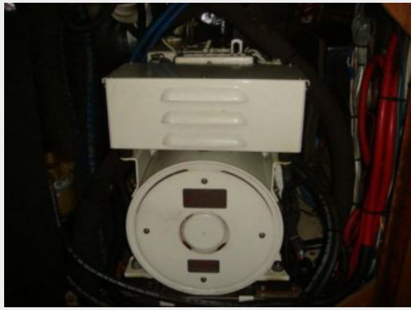
42' Hunter generator photo2
