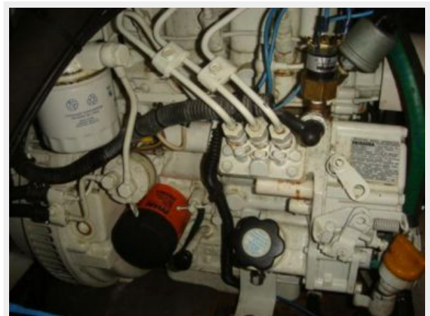
42' Hunter generator photo1
