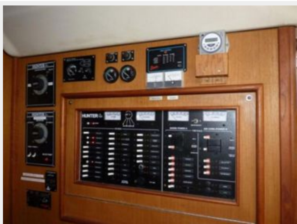
42' Hunter electrical panel
