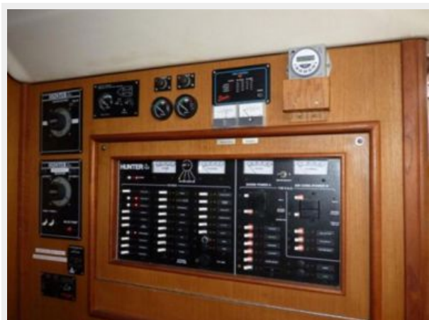
42' Hunter electrical panel
