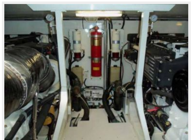
Engine Room Looking Forward
