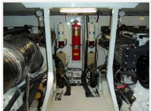
Engine Room Looking Forward
