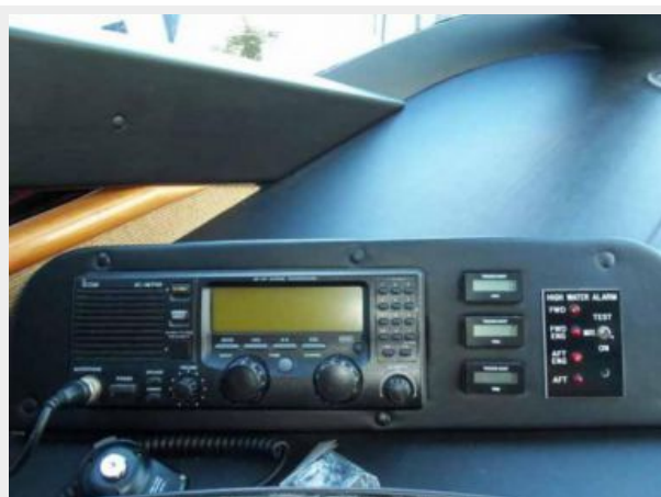
Salon SSB & Bilge Alarm
