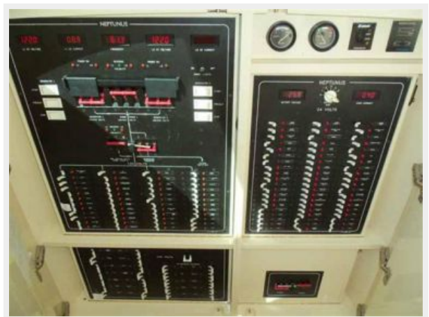
Companionway Electrical Panel
