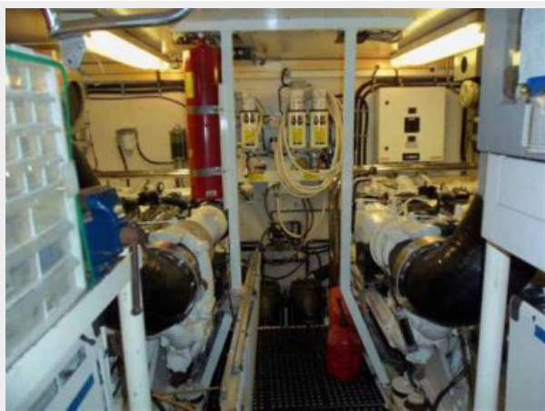
Engine Room Looking Forward
