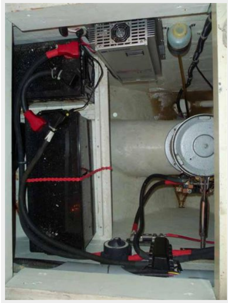
VIP Thruster, Batteries & Charger
