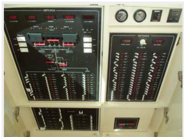
Companionway Electrical Panel
