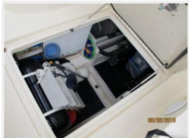
Large Engine Room
