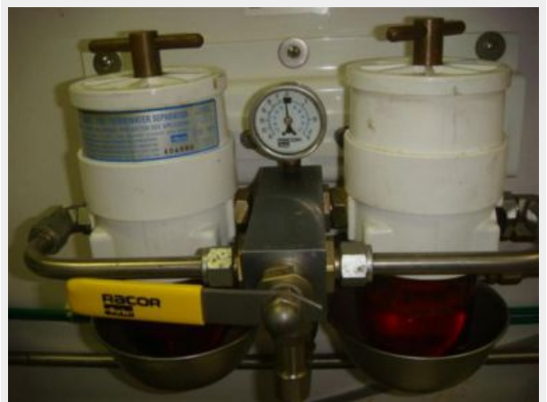
67' Lyman-Morse starboard generator Racor fuel filters
