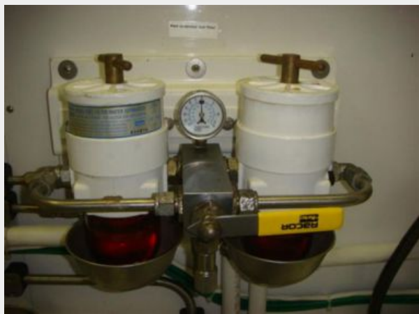
67' Lyman-Morse port generator Racor fuel filters
