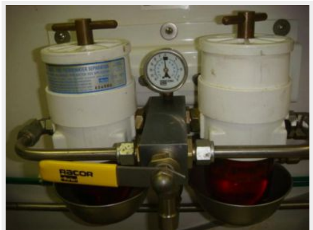
67' Lyman-Morse starboard generator Racor fuel filters
