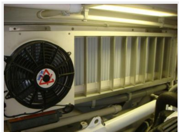
67' Lyman-Morse engine room Delta-T air filtration system
