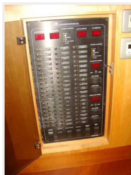
67' Lyman-Morse pilothouse electrical panel
