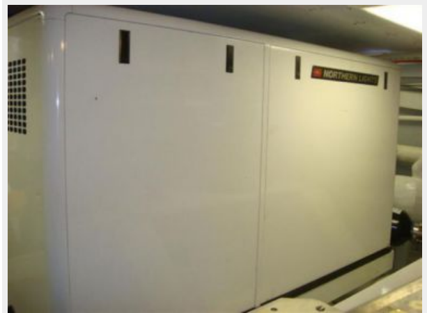
67' Lyman-Morse starboard generator sound box
