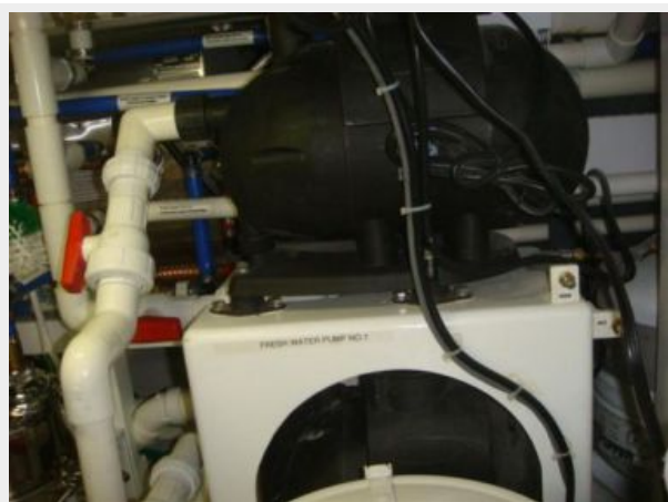
67' Lyman-Morse fresh water system pumps
