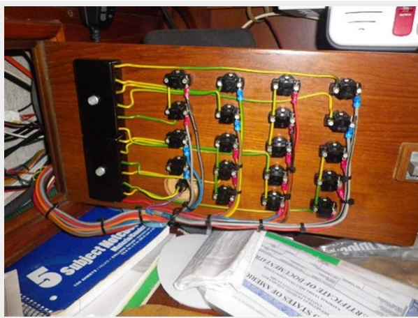
Breakers for 12volt electrical
