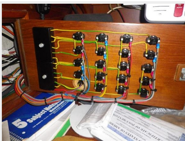
Breakers for 12volt electrical
