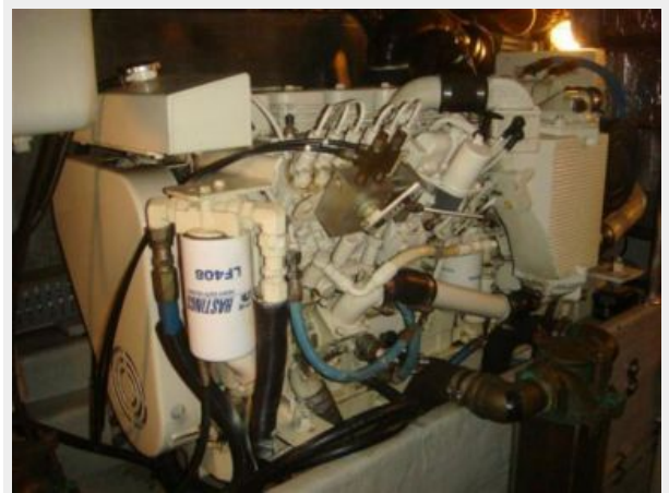
43' Mainship starboard main engine
