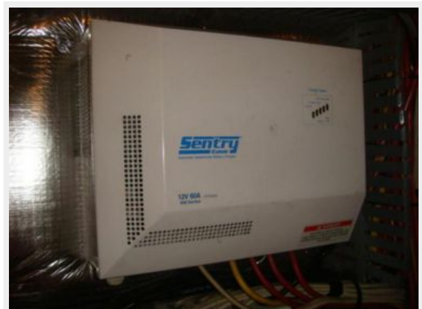
43' Mainship battery charger
