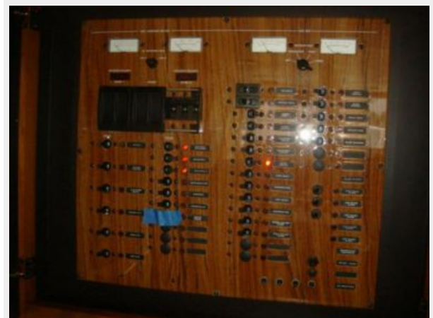
43' Mainship electrical panel
