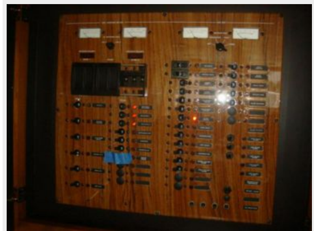
43' Mainship electrical panel
