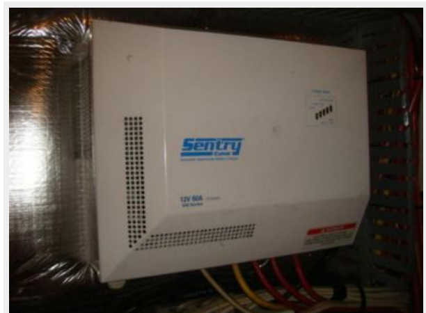
43' Mainship battery charger
