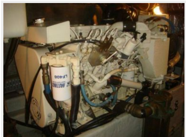
43' Mainship starboard main engine
