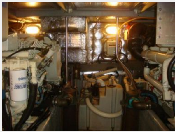
43' Mainship engine room
