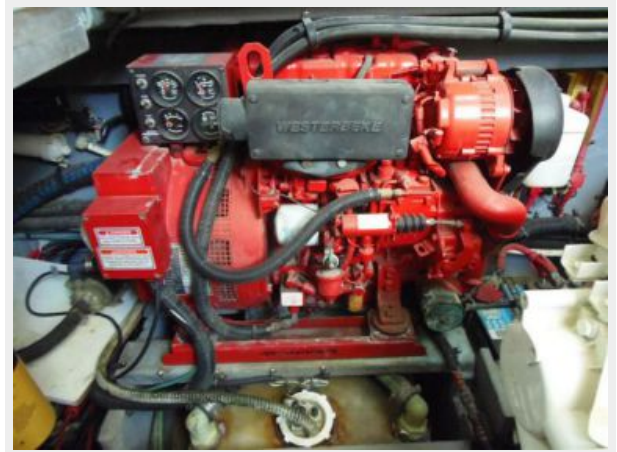
Sea Ray 370 aft cabin genset
