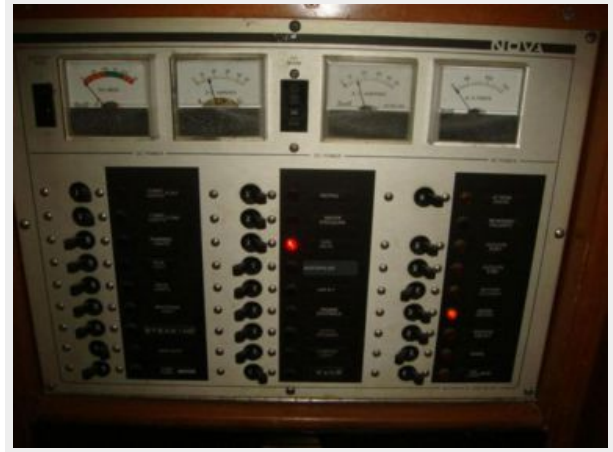
38' Cabo Rico electrical panel
