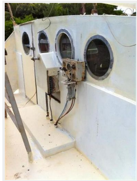
engine controls forward of helm
