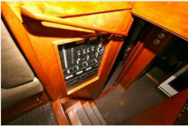
MAIN ELECTRIC PANEL
