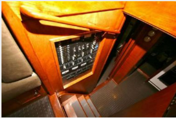
MAIN ELECTRIC PANEL
