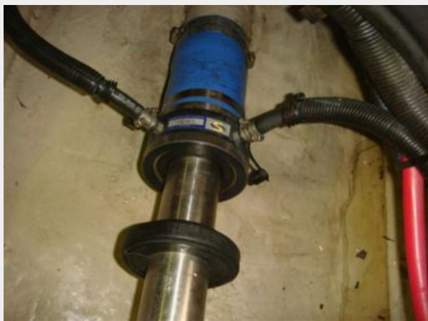
54' Sea Ray starboard shaft seal
