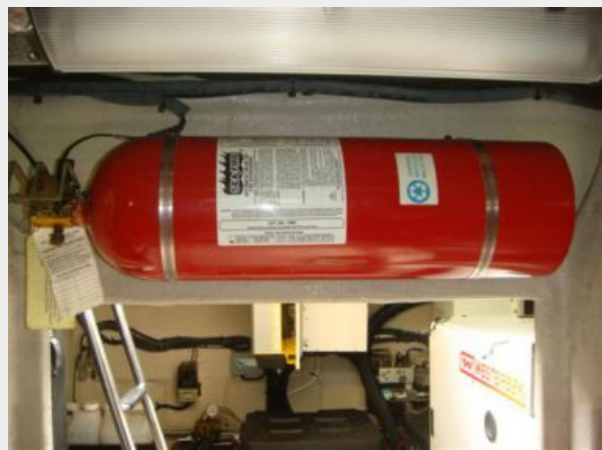
54' Sea Ray fire suppression system
