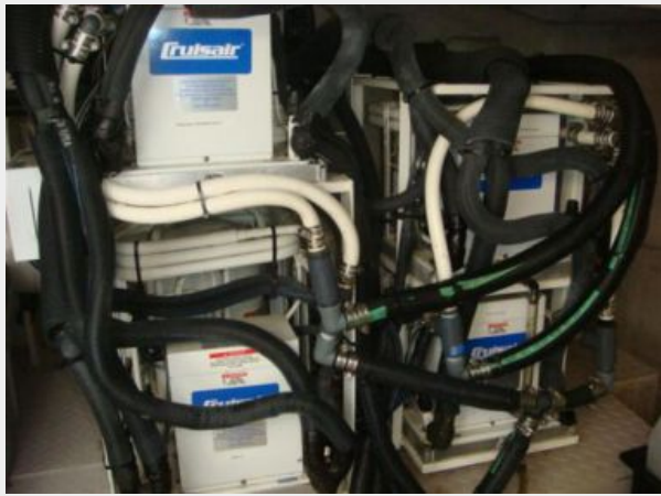
54' Sea Ray air conditioning system
