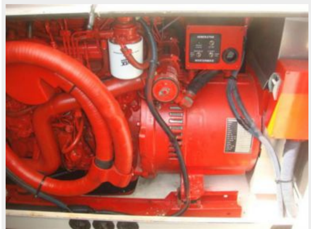
54' Sea Ray generator
