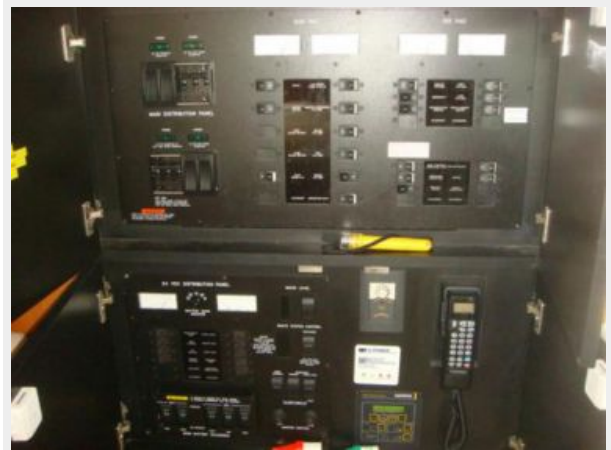
54' Sea Ray electrical panel
