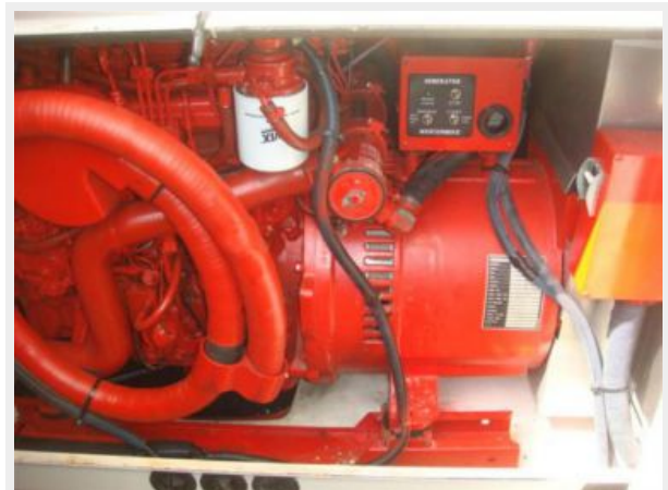
54' Sea Ray generator
