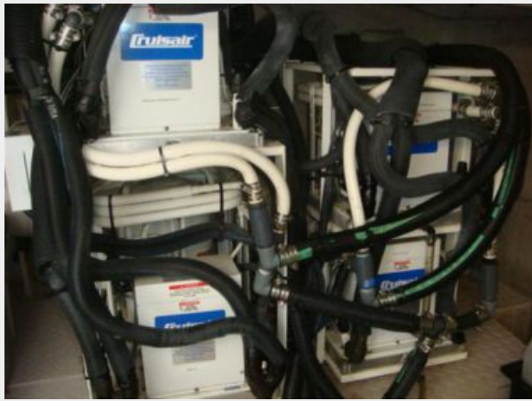
54' Sea Ray air conditioning system
