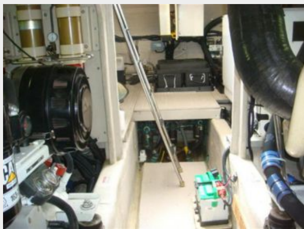
54' Sea Ray engine room aft
