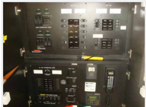
54' Sea Ray electrical panel
