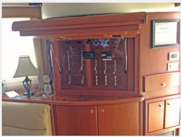
ELECTRICAL PANEL AFT OF DINETTE
