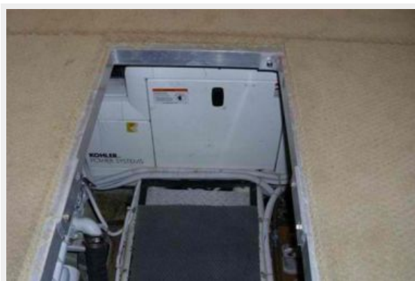
Kohler Generator in Sound Shield
