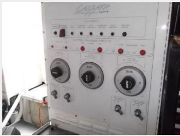
DC Battery Panel
