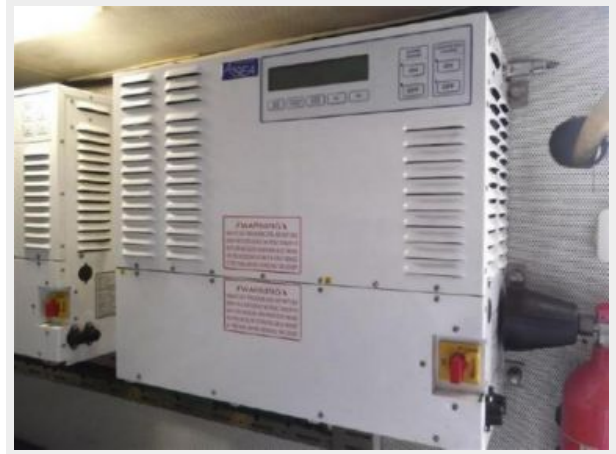
12 KW Shore Power Converters
