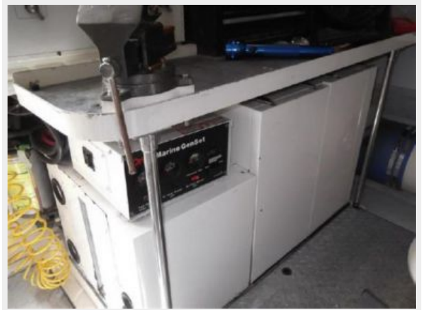
Port Onan Generator
