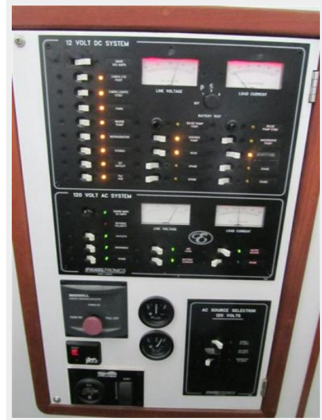
36' Endeavour electrical panel
