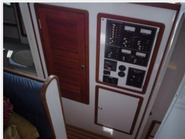
36' Endeavour storage/electrical panel
