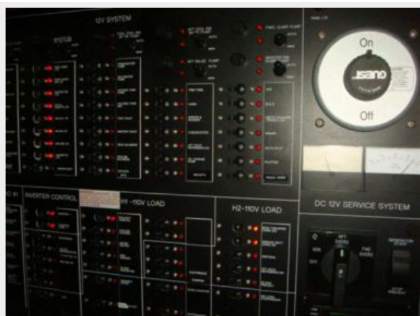
55' Ocean Alexander electrical panel
