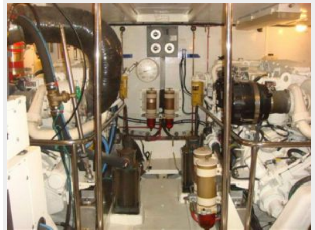
55' Ocean Alexander engine room forward
