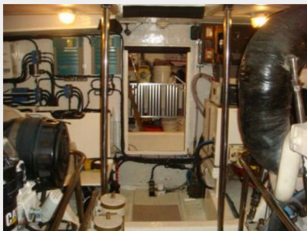
55' Ocean Alexander engine room aft
