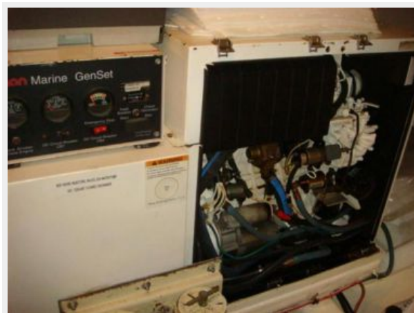
55' Ocean Alexander generator
