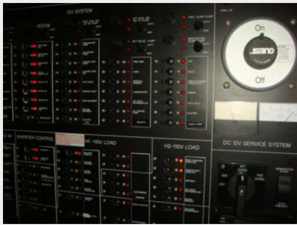
55' Ocean Alexander electrical panel
