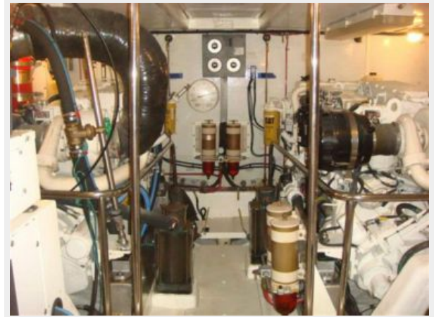
55' Ocean Alexander engine room forward
