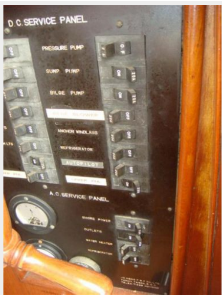
36' Albin electrical panel
