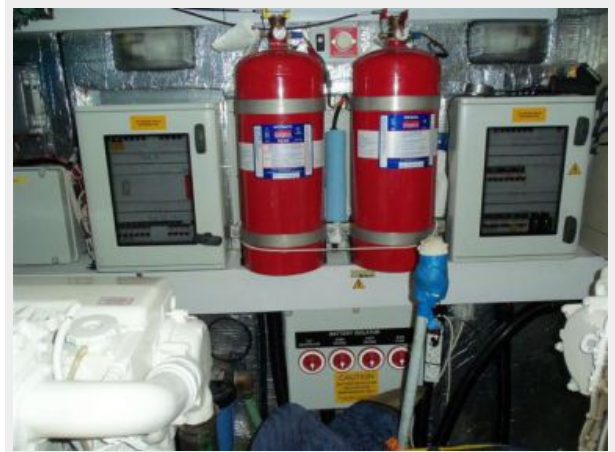
Engine Room Looking Aft
