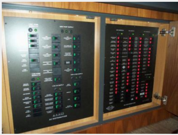
Helm Electrical Panel
