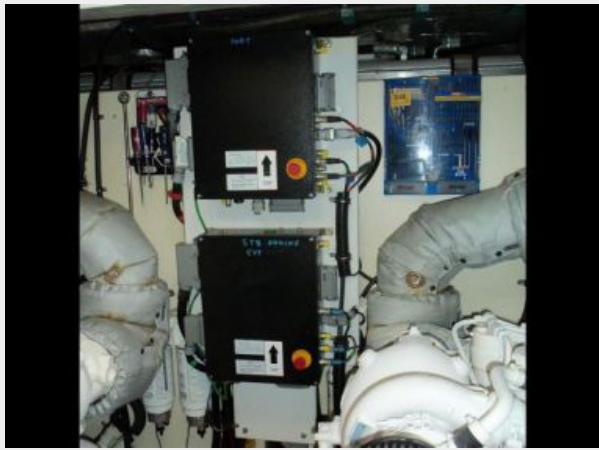
Engine Room Looking Forward
