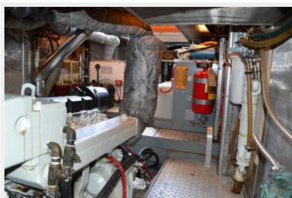
Nordhavn 40' Engine room
