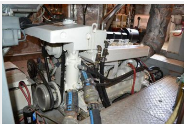
Nordhavn 40' Engine room
