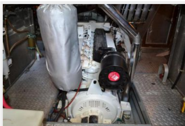
Nordhavn 40' Engine room
