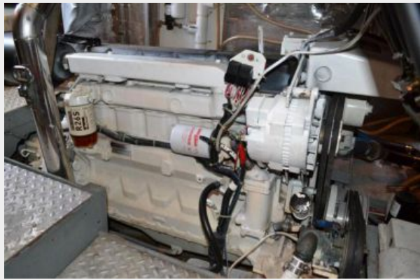
Nordhavn 40' Engine room
