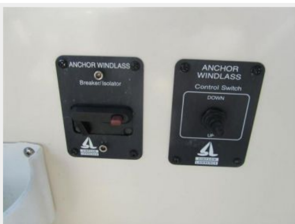
Rinker 310 Windlass breaker & helm controls
