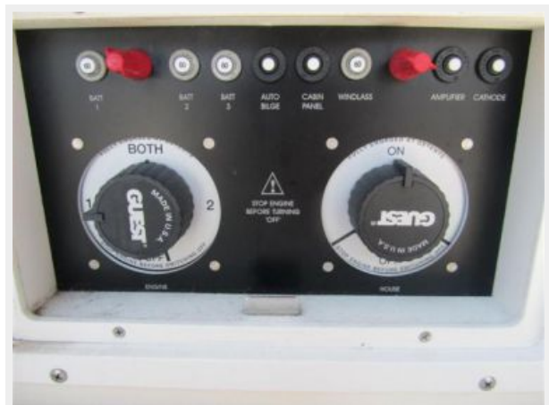
Rinker 310 Battery selector switches
