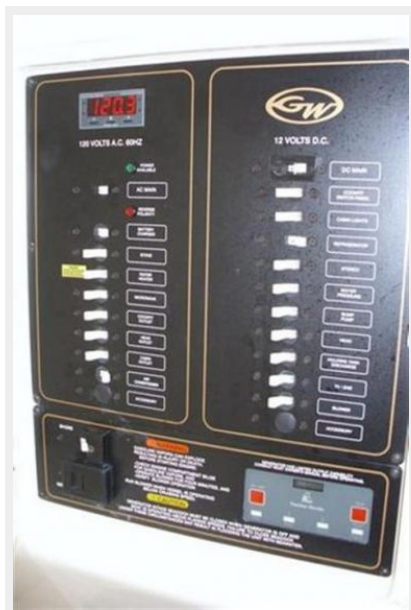
Grady White Electrical Panel
