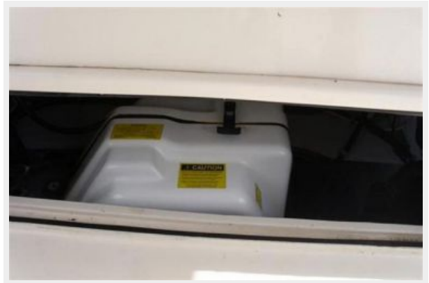
Panda 4Kw Diesel Generator In Sound Shield
