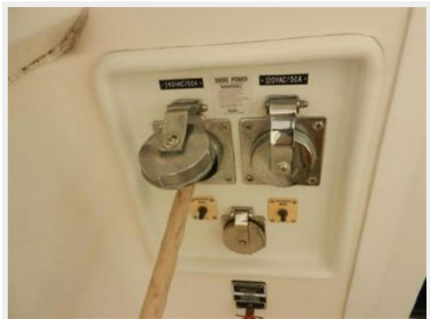
Dual Automatic Shorepower Cable Masters/Controls
