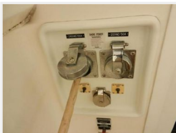
Dual Automatic Shorepower Cable Masters/Controls
