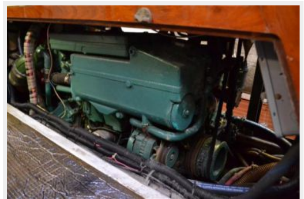
58' Farr Custom Engine- port side
