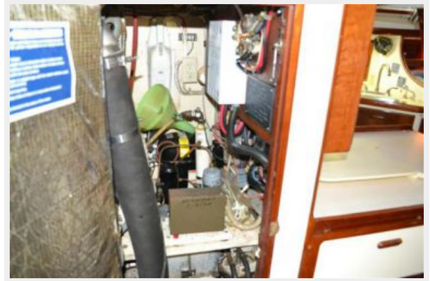
58' Farr Custom Charger/Inverter closet
