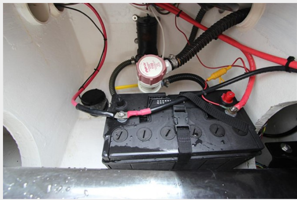
Port Side Battery Compartment
