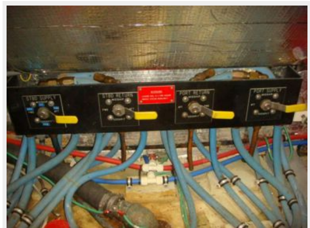
52' Hatteras fuel manifold
