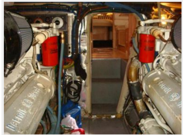
52' Hatteras engine room forward
