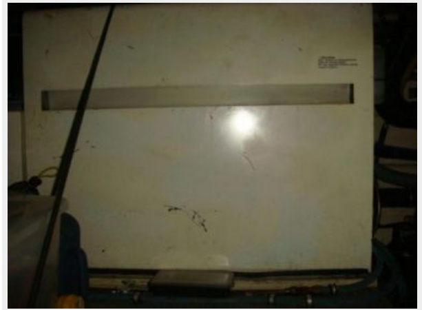
52' Hatteras generator sound box
