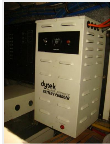
52' Hatteras battery charger
