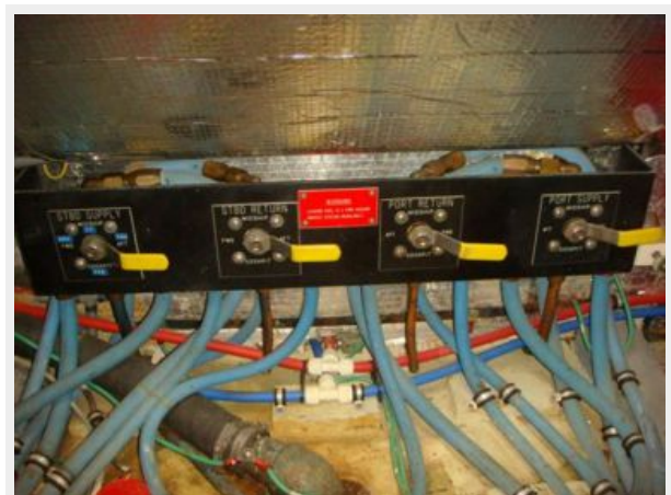
52' Hatteras fuel manifold
