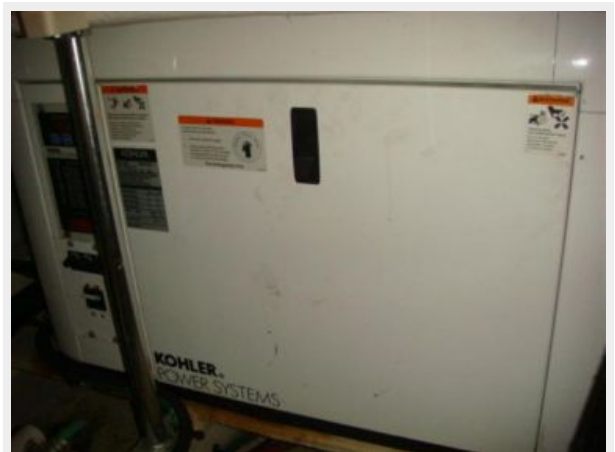
40' Mainship generator sound box
