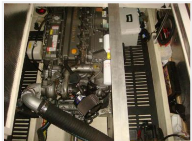
40' Mainship engine room
