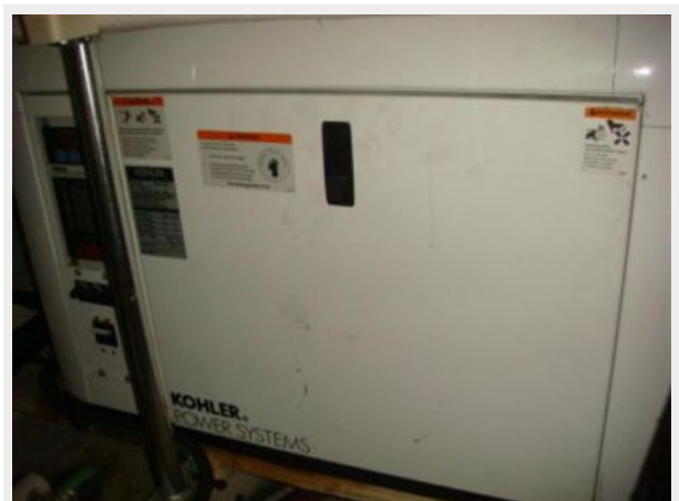
40' Mainship generator sound box
