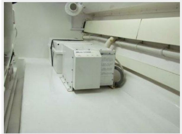
Outboard of Stbd Engine & Charles Shore Power Transformers
