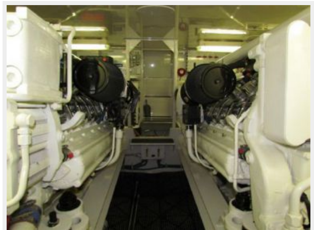
Engine Room Looking Aft
