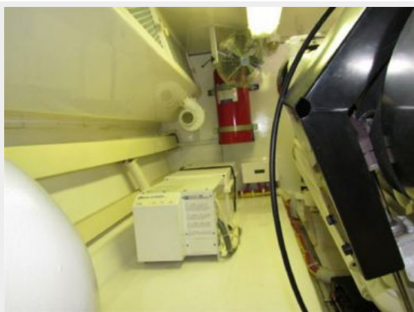
Outboard Port Engine & Charles Shore Power Transformer
