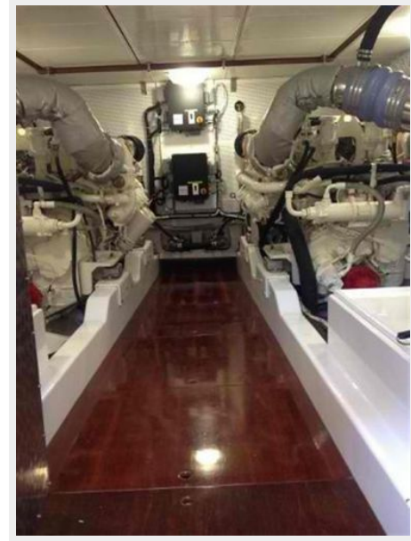
Engine Room View
