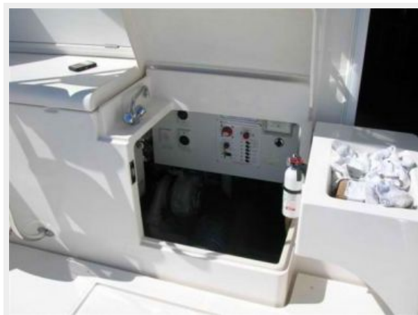
Engine Room Access
