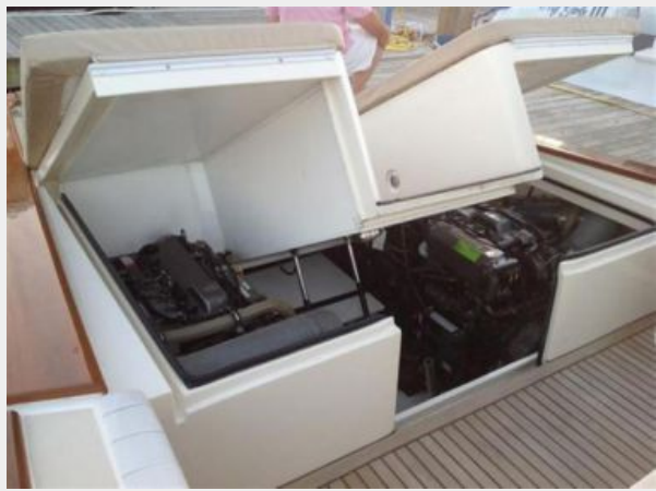
Electric Engine Hatch
