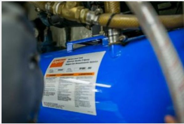
Engine room - fresh water system
