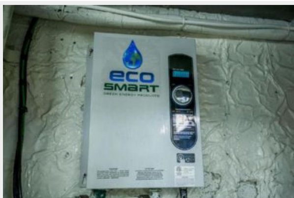
Engine room - eco smart hot water heater
