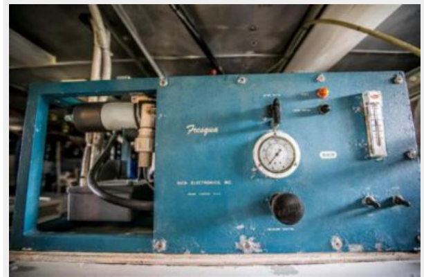
Engine room - water maker
