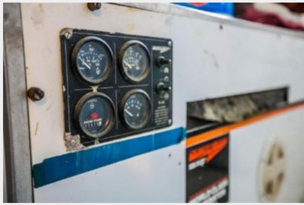
Engine room - 20 kw Northern Lights GenSet
