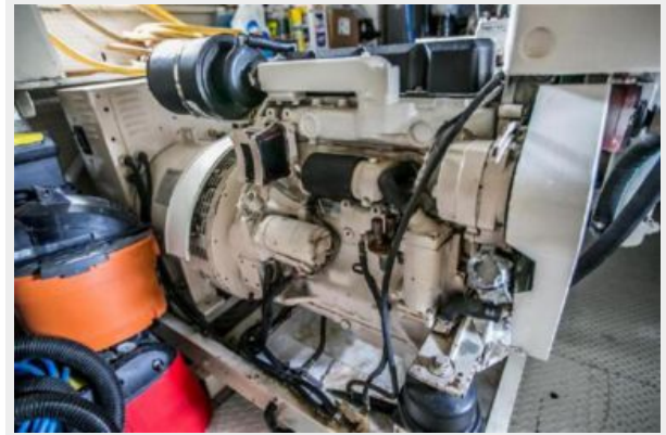
Engine room - 30kw Northern Lights GenSet
