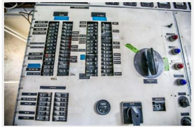
Engine room - control panel
