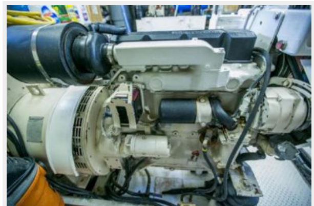
Engine room - 30kw Northern Lights GenSet
