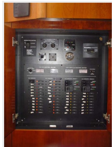
Electrical Panel in Salon Portside Cabinetry
