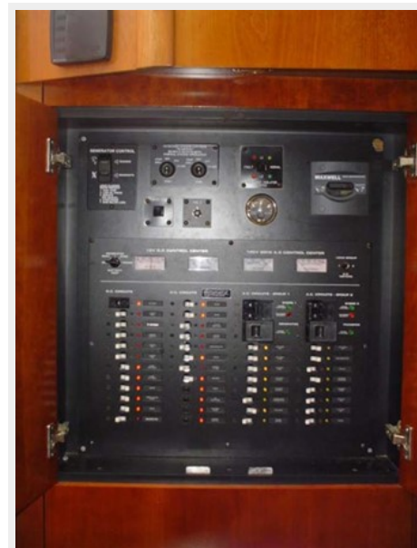
Electrical Panel in Salon Portside Cabinetry
