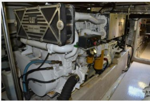
56' Sea Ray Engine room
