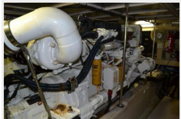
56' Sea Ray Engine room
