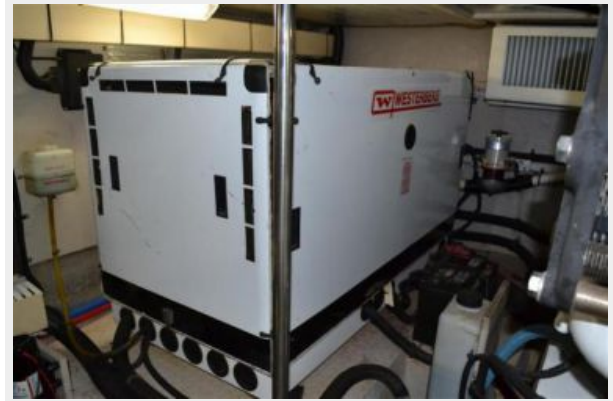
56' Sea Ray 20KW Generator
