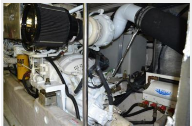
56' Sea Ray Engine room
