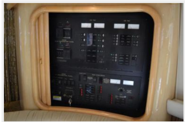
56' Sea Ray Electrical Panel
