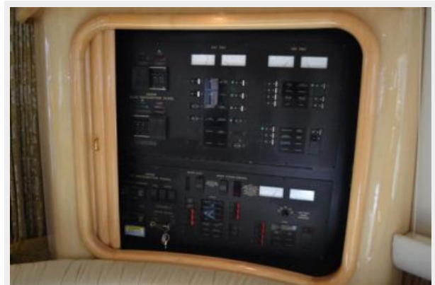
56' Sea Ray Electrical Panel
