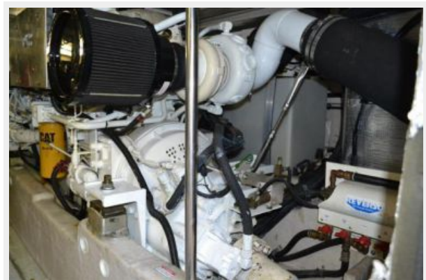
56' Sea Ray Engine room
