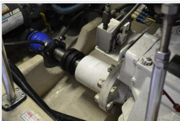
56' Sea Ray Engine room
