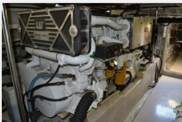
56' Sea Ray Engine room
