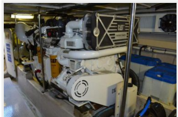
56' Sea Ray Engine room
